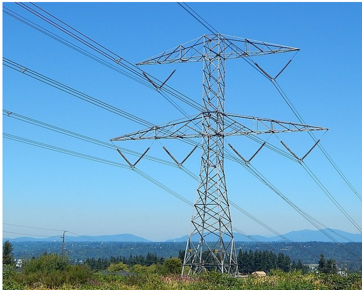
High Voltage Transmission Tower and Lines. Auburn WA, (Credit: Ron Clausen, Wikimedia Commons author (GNU Free Documentation License - public domain) [32])
