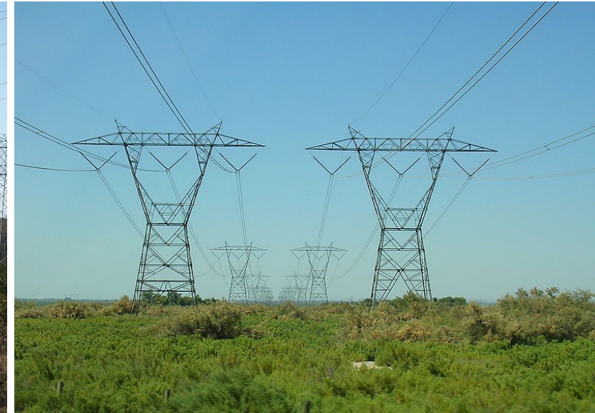
Close View of a 500kV Lines, Southern California Edison's Path 26 (Credit: Raumfahrt Hauptfokus (Henristosch), Wikimedia Commons author (GNU Free Documentation License - public domain) [33])
