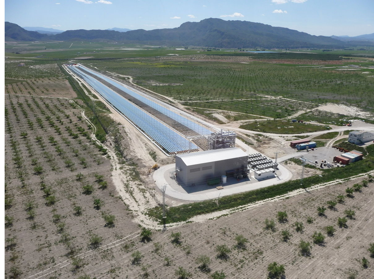
Figure 6-5: Linear Fresnel reflectors.
