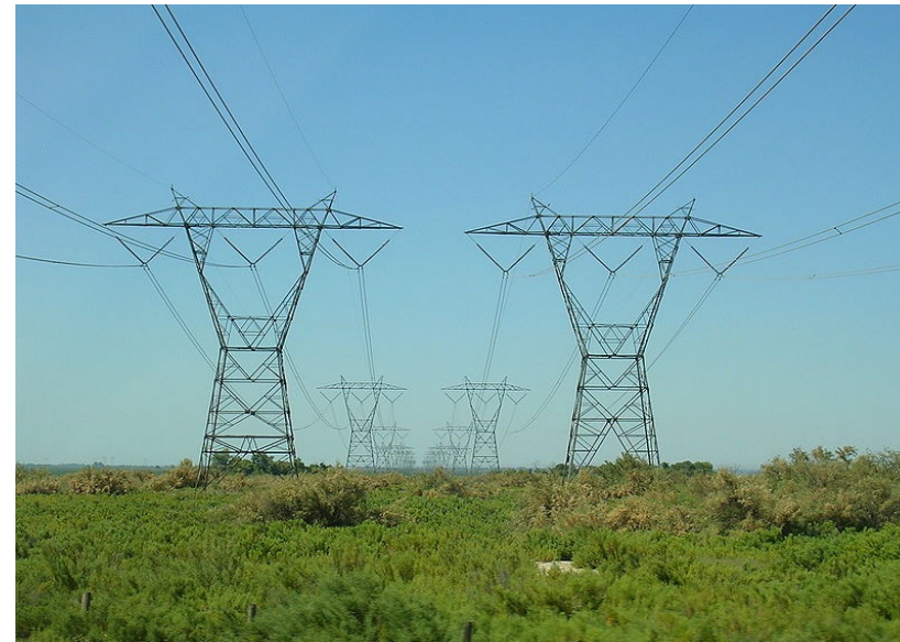
Close View of a 500kV Lines, Southern California Edison's Path 26 (Credit: Raumfahrt Hauptfokus (Henristosch), Wikimedia Commons author (GNU Free Documentation License - public domain) [33])
